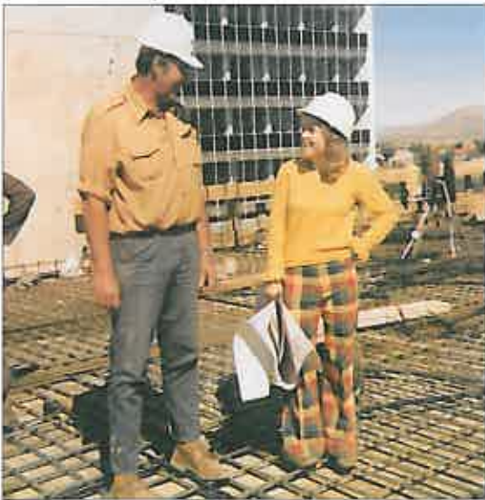
Allyson on site in Windhoek in her Ove Arup days discussing 'reinforcing of concrete' with site foreman Alex Reyneke
